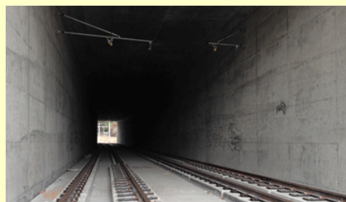
4. Looking east into the same tunnel after the first graffiti removal and after track and the overhead catenary system (OCS) supports were installed. Notice in the photo that the graffiti was starting to reappear.
