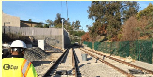
2. Looking west toward the tunnel under the I-10 (Santa Monica) Freeway just east of Overland Boulevard in West Los Angeles. This former single track freight tunnel was found to be wide enough for a two track LRV line. Seen in the photo is George Flowers of the Construction Authority. This is not far from the location where the original Palms Depot was once located.
