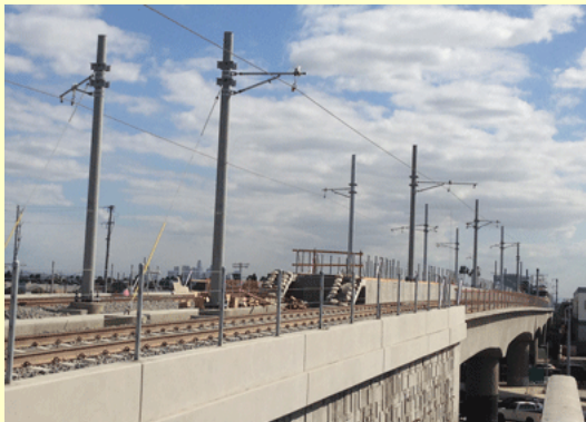
1. Looking east at the new bridge at Venice & Robertson. You can see a train at the station inn the distance almost ready to return to Los Angeles.
