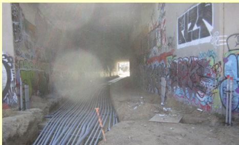
3. Looking west into the tunnel under the I-10 freeway. This is before the graffiti was removed (the first time). All under track conduits were installed before foundation for track was poured.
