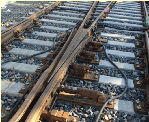
8. A spring frog used on all four switches at Military interlocking. Note the concrete ties now used under the switches.
